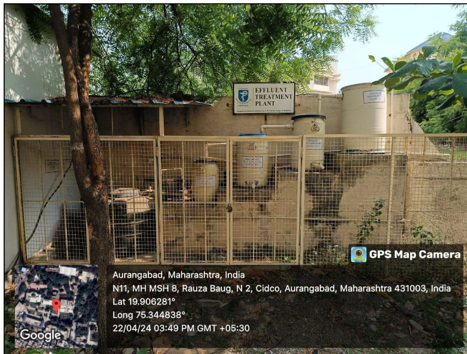
Effluent Treatment Plant for treating waste Water generated from college and its laboratory before releasing to sewage
