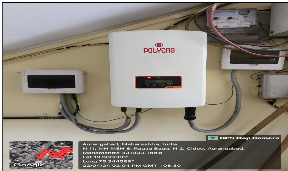
Inverter (Wheeling Grid) is a part of solar panel system
