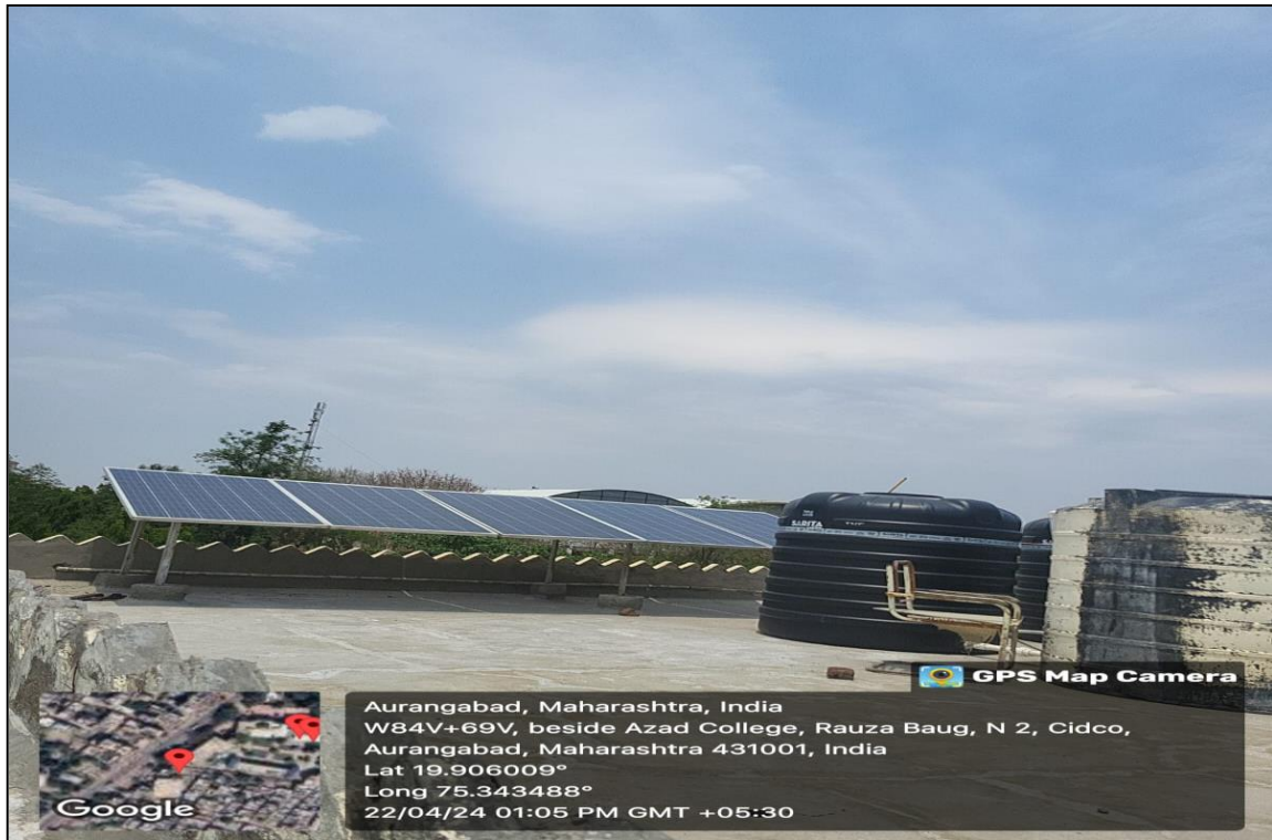
Installed Solar Panel (PV cell) at Institute Roof with capacity of 10KW
